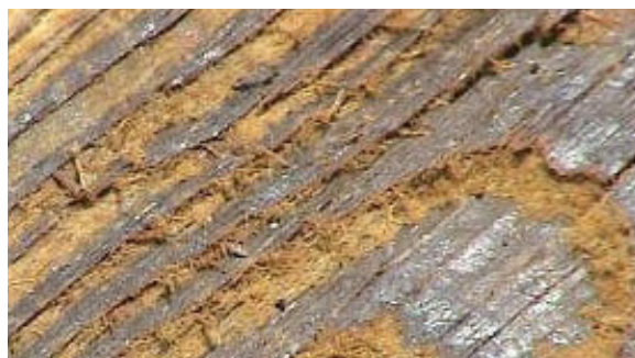
Wood damaged by pressure washing
